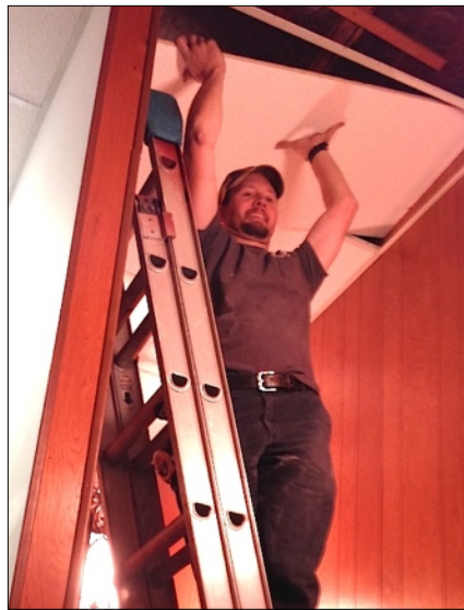
Nov 20, 2014 — Salem Trustee, Brandon Leatherman helps install new ceiling tiles in the hallway of the educational building.
